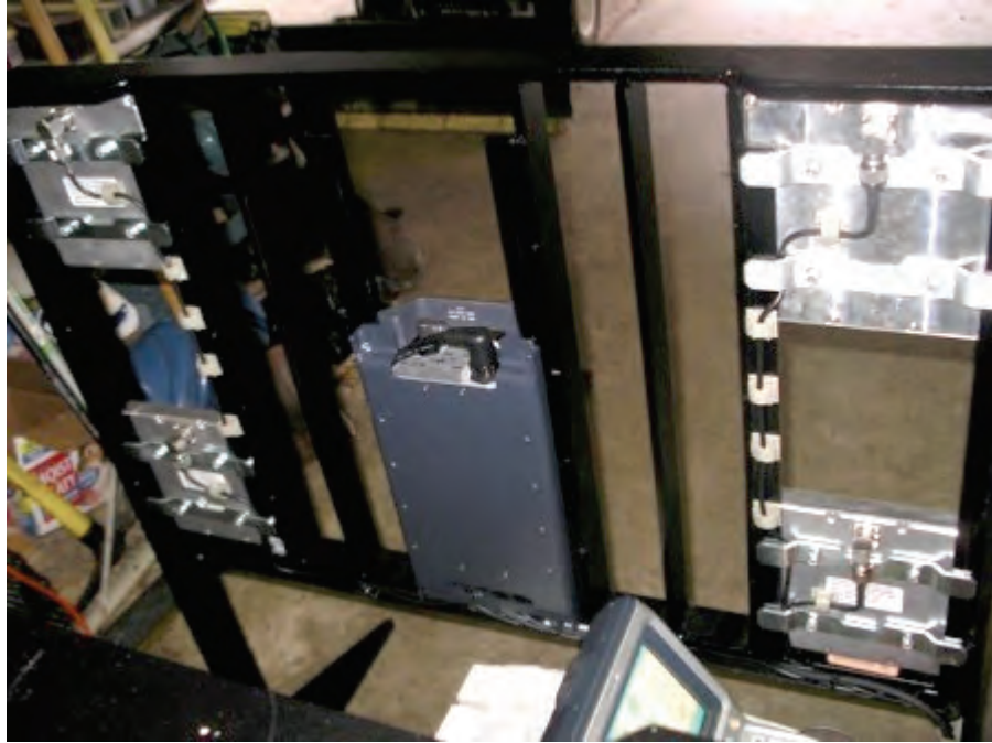
Backside of ALBR: Note cable tiedowns along ALBR rails. All cables are run to cable tray for added protection.
