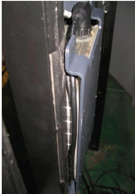
Close-up of Cable Routing: Note cables run down along rails to cable tray below.
